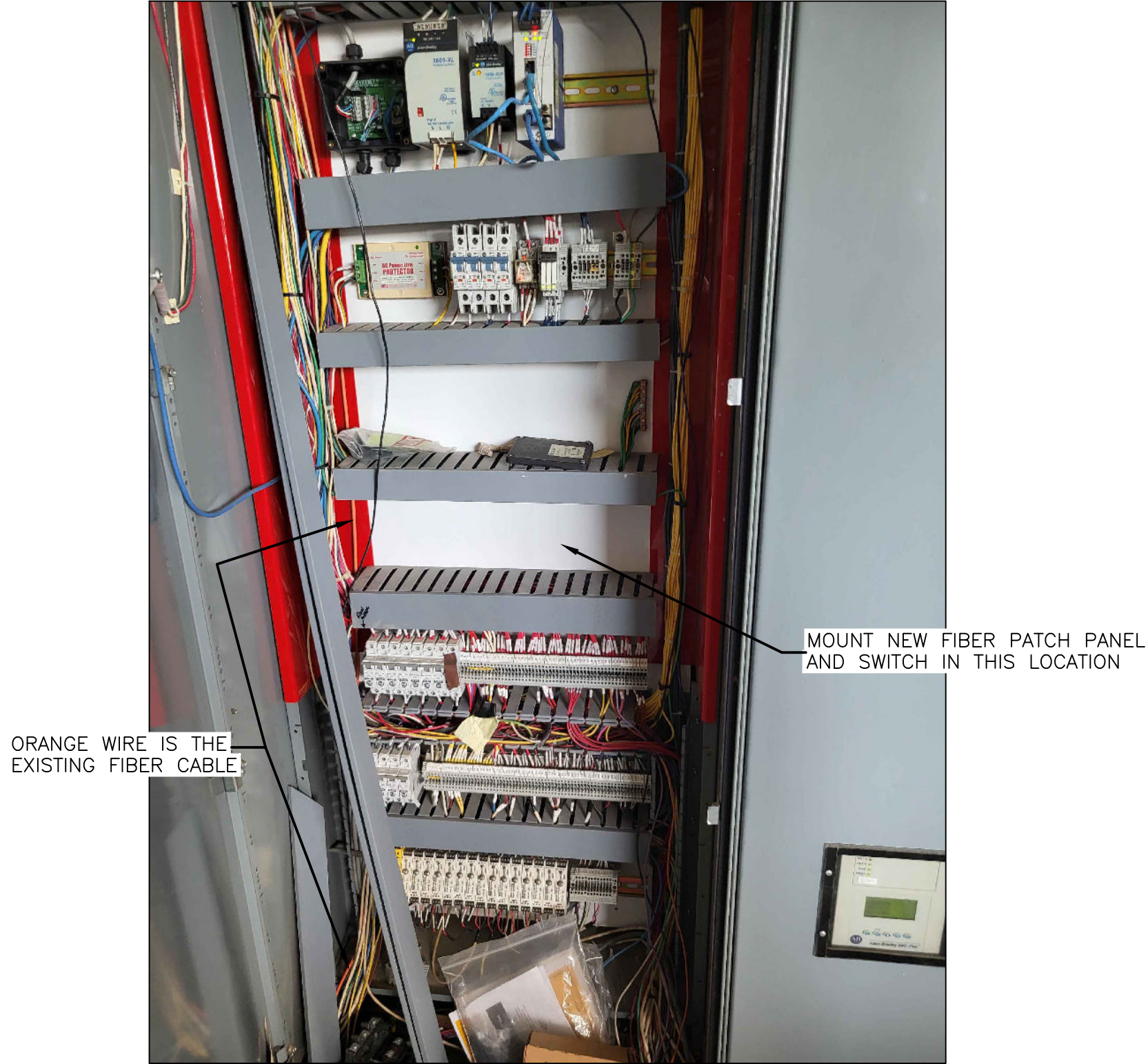
CONTROL PANEL 2 CONTROL SECTION IN LOAD CENTER 1
