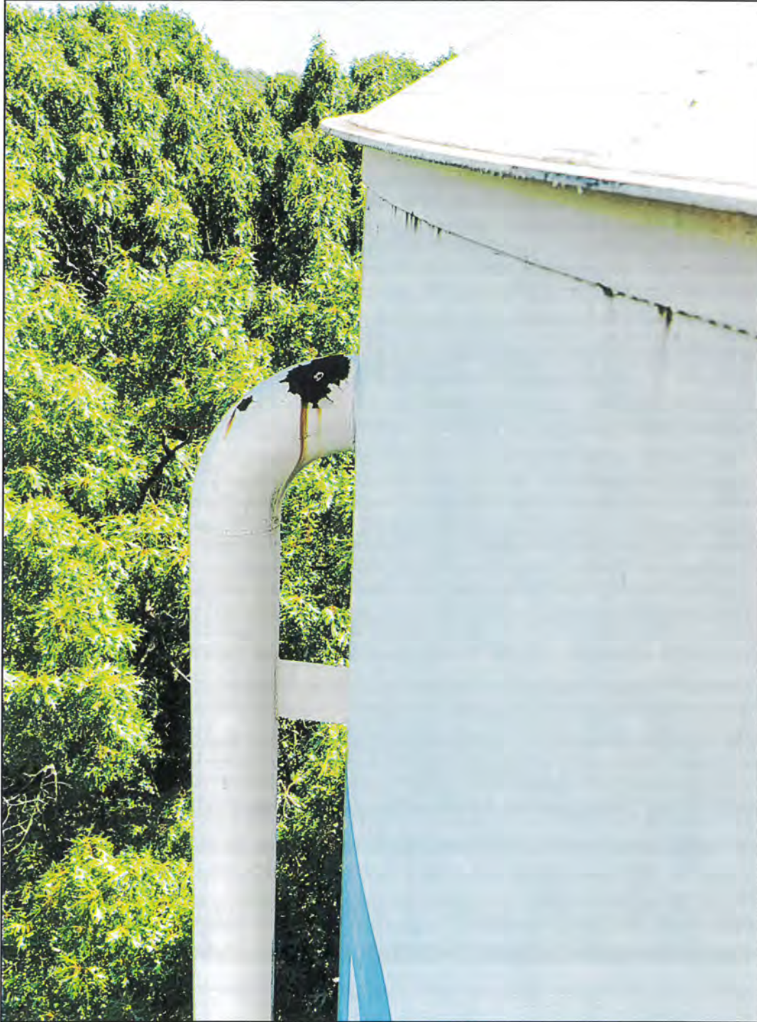
DAMAGE TO OVERFLOW PIPE
