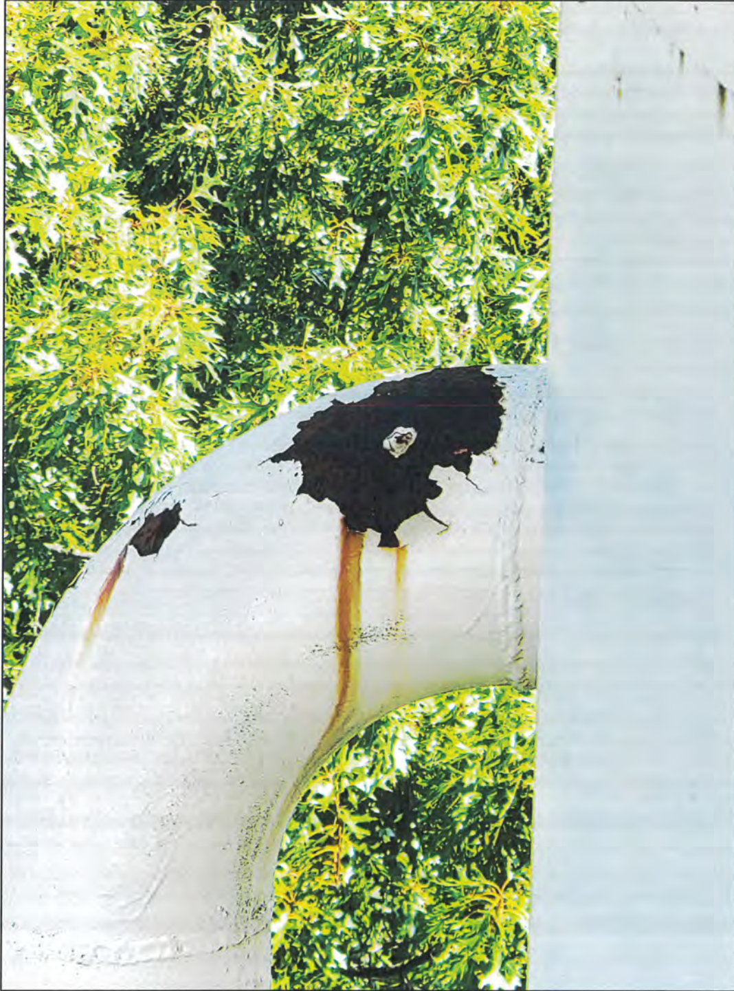
CLOSE UP OF DAMAGE TO OVERFLOW PIPE
