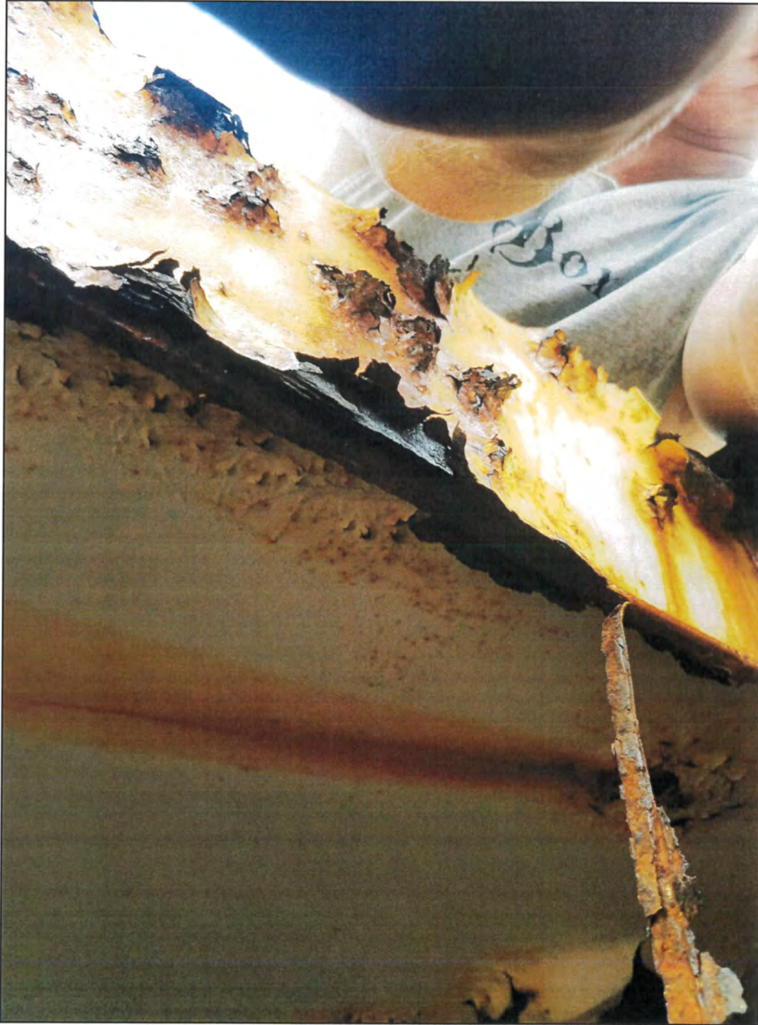
INSIDE OF ACCESS HATCH
