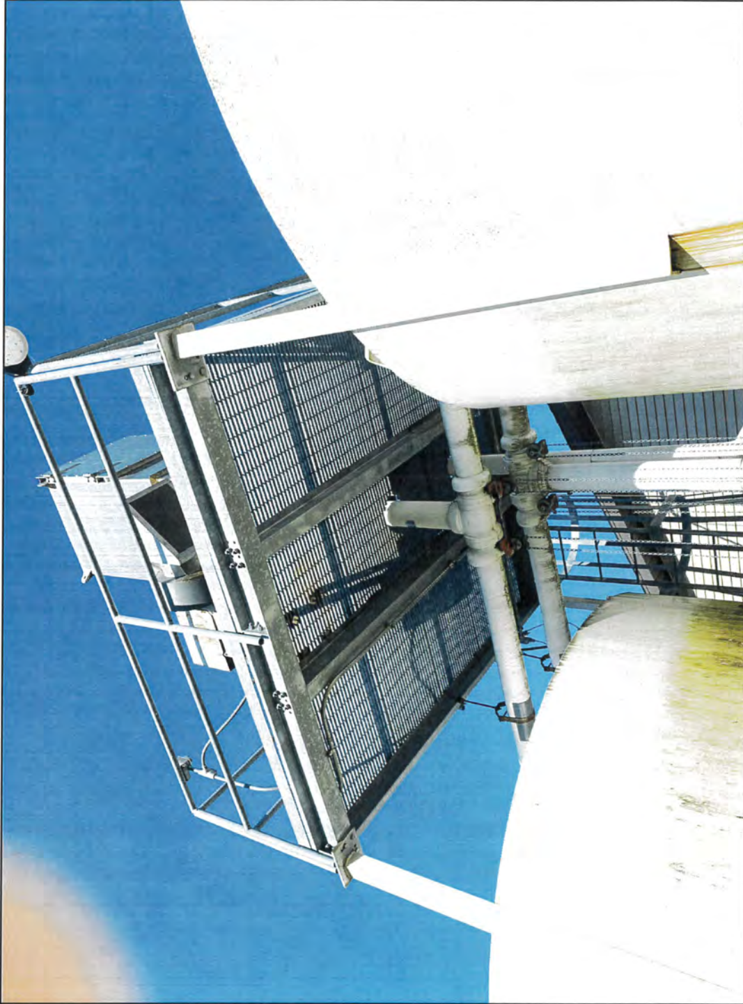
AERATOR ABOVE TANKS
